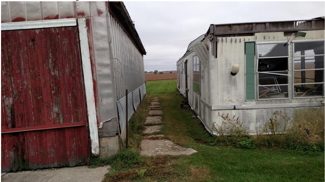
Figure 6 Looking at the separation between the old mobile home and the barn
